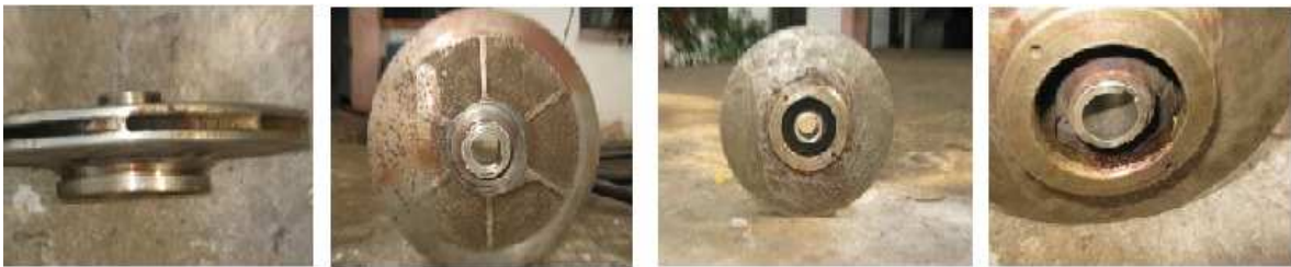
Figure 23: Impeller Damage Due to Cavitation Erosion
